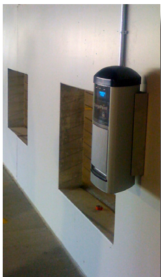
Charging Station in Downtown Nashville's Fulton Parking Garage
